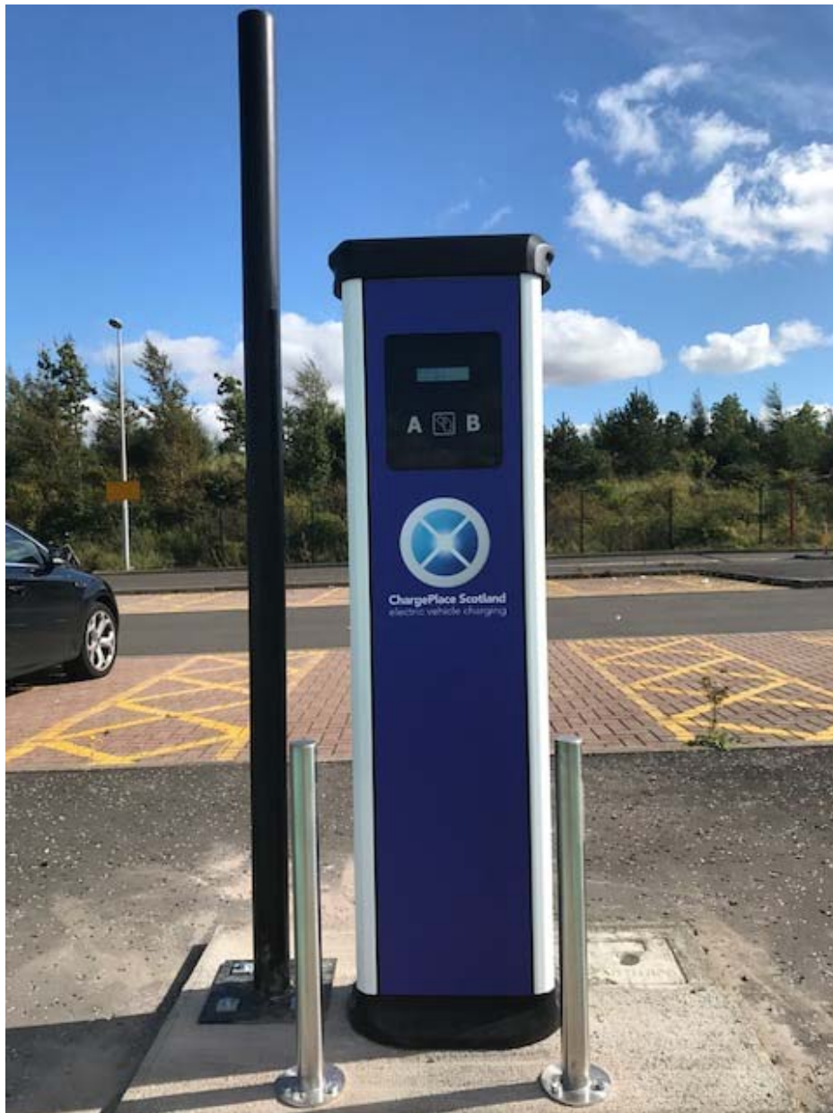
EV charging unit, Straiton Park and Ride, Edinburgh
