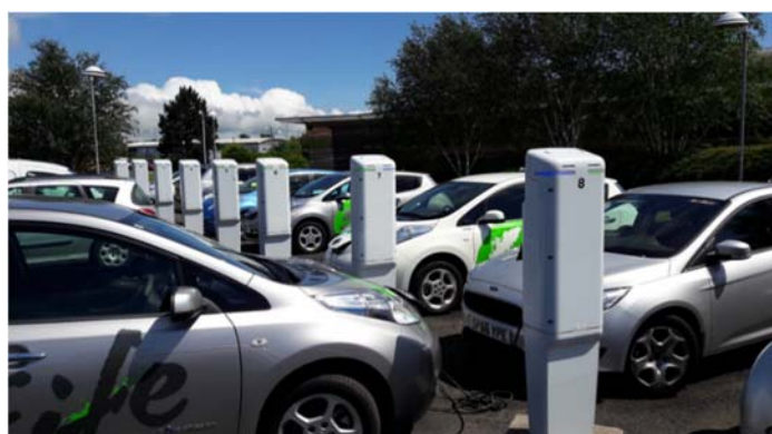
Example of an EV charging hub (APT Controls)
